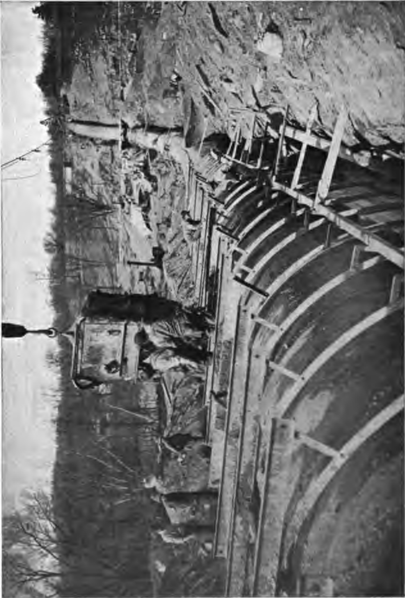
PLATE 154.—Contract 68. Placing Outer-lining of Steel Pipe Siphon. Outside forms, steel ribs with wooden lagging. Concreting done while pipe is filled with water under working pressure.
